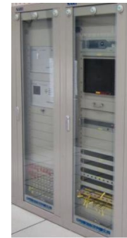
Fig.6 Photo of control & protection system cabinet of SVG
