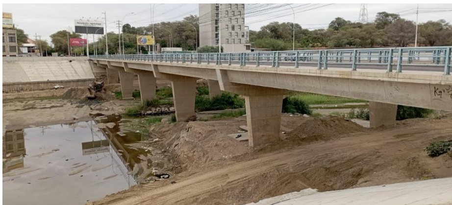
Fig. 1. Condition of the piers of the Andrés Avelino Cáceres bridge.
