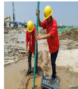
Figure 3. PVC water level tube
