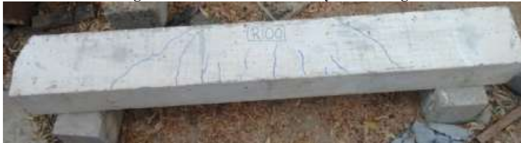
Figure 4.15 R100 beam after cyclic loading
