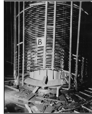
Fig. 8. Photo of phase “B” of the low voltage winding of 250MVA / 220 kV transformer, illustrating the loss of the axial stability of the winding, i.e. the movement of the winding in the axial (vertical) direction under the action of electrodynamic forces during the flow of short-circuit currents.
