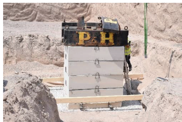
Fig. 9. View of the elements used for the application of the test load.
