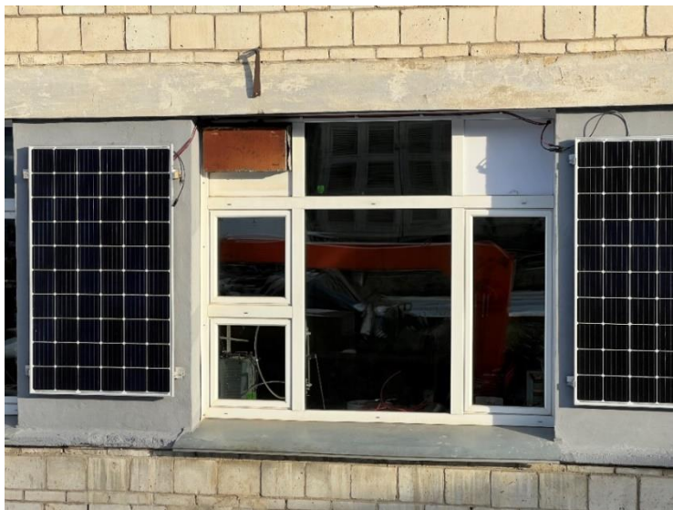
Fig. 2. Appearance of photovoltaic converter.
