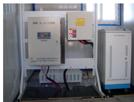
Fig.5 Site photos of controller and inverter
