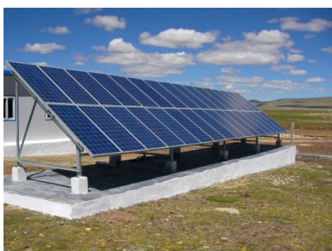
Fig.3 Site photo of solar photovoltaic array
