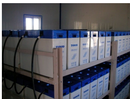
Fig.6 Site photo of battery pack
