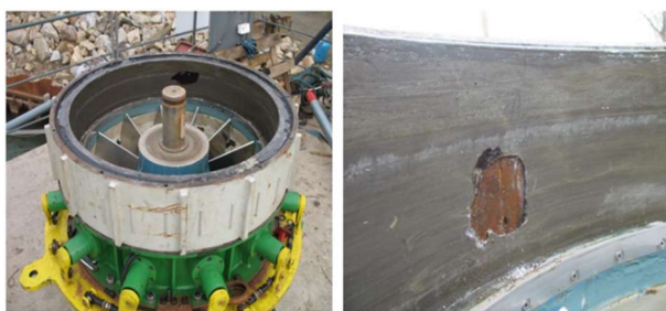
Fig. 9. Burnout of the stator insulation due to an electrical short circuit resulting from poor electrical insulation in the turbine integrated in the wet gap.
