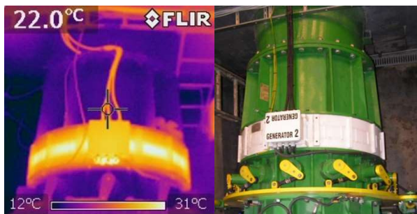
Fig. 6 Temperature distribution of the stator of the integrated hydro unit (the stator temperature at rated load did not exceed 36 °C)
