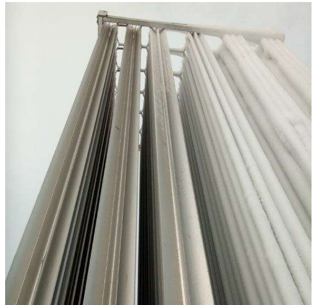
Fig. 1. Longitudinal finned tubes with accumulated ice.
