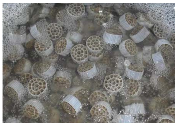
Fig. 3. MBBR biochemical pool in operation.
