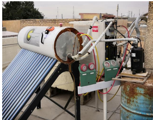
Fig. 4. The outdoor unit integrated with the solar collector.
