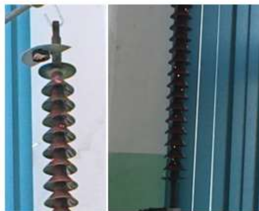
Fig. 5. The picture of the discharge activity on the insulator with pollution in the laboratory [14].
