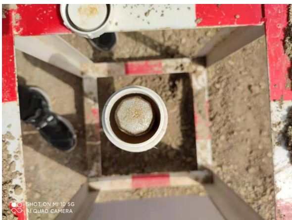
Picture 2 Settlement detection device
