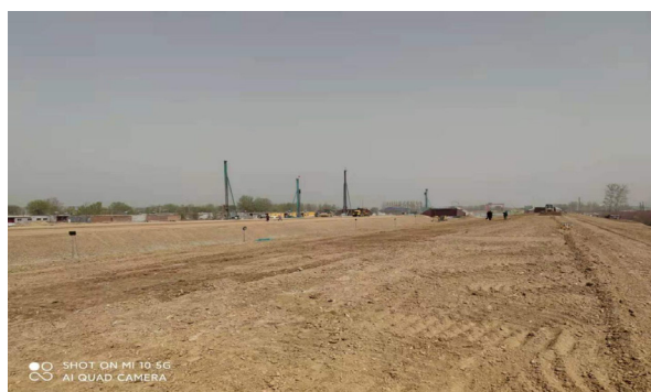
Picture 1 Settlement detection device
