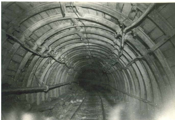
Fig. 8. An example of good stability of a roadway driven in compacted and consolidated goaf.
