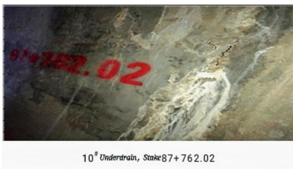
Figure 3 Cracks in expansion joints of Hejiacha culvert
