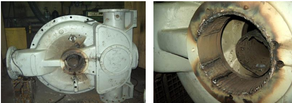
Fig. 3. Depreciation of the working bodies of the centrifugal pump PS "Charkhin"
