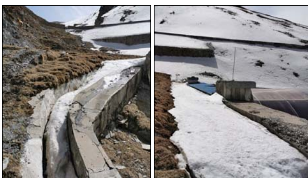
Fig. 4. Freezing of Roof Intercepting Ditches.
