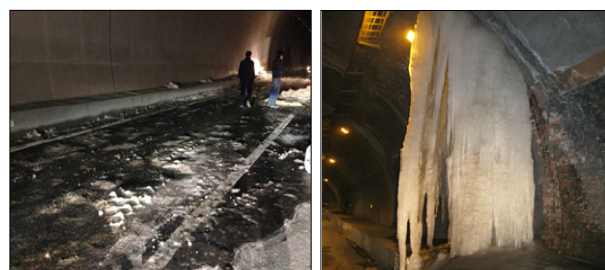
Fig. 2. Pavement Icing and Ice Covering on Lining in Tunnel.
