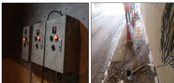
Fig. 9. Electric Tracing Heating System .
