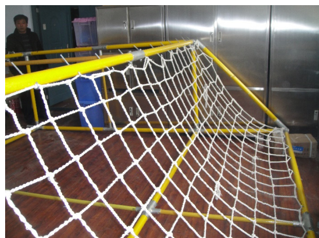
Fig. 4. Insulation protection frame protection net physical picture
