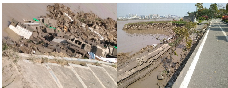
Fig.1 Collapsed marine embankment in-situ
