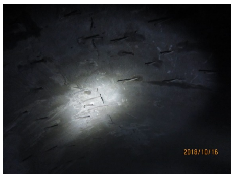
Fig. 5 Spalling of Sprayed Concrete
