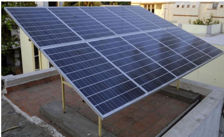
Figure 9: Roof top Solar Power heater and plant
