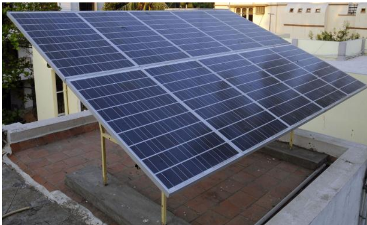
Figure 9: Roof top Solar Power heater and plant
