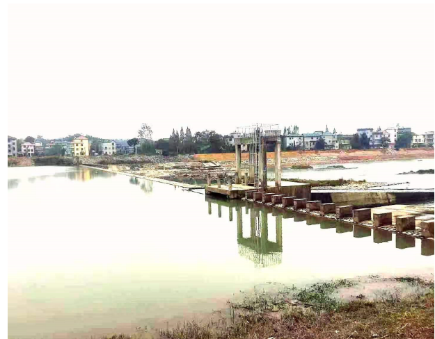
Fig 1. Leakage at the intake
