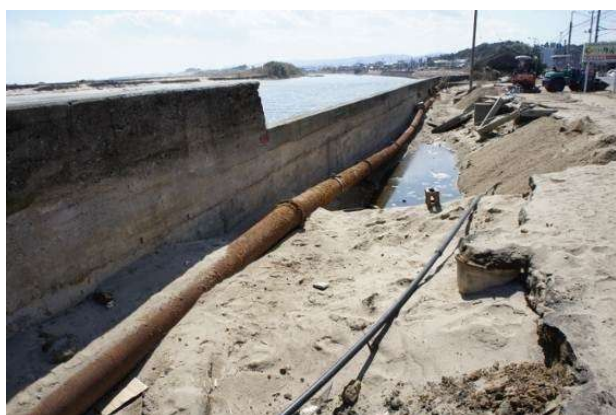
Fig. 9. Damaged pipe behind a seawall
