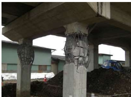
Fig. 23. Damaged viaduct columns of the Tohoku Shinkansen line after the Tohoku earthquake (photo courtesy of Dr. Takahashi, DPRI, Kyoto Univ.)
