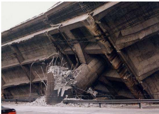
Fig. 2. Collapsed pillar of a highway viaduct caused by shear failure
