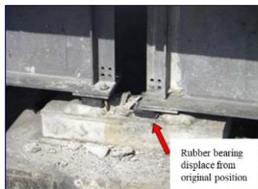
Fig. 12. Damages of bridge deck due to the displacement of rubber bearing post-Padang Earthquake in 2009 [27]
