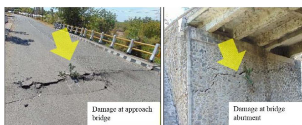
Fig. 13. Damages of bridge deck due to compression effect in longitudinal direction post-Nusa Tenggara Barat Earthquake in 2018 [27]
