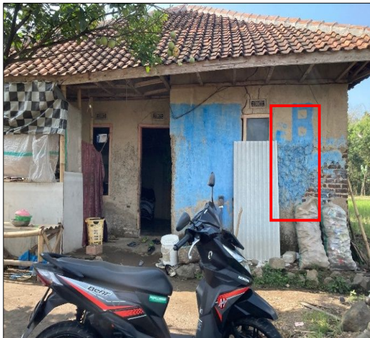
Fig. 4. A building located at CPTu-04. It has a wide crack opened and was marked inside a red box.
