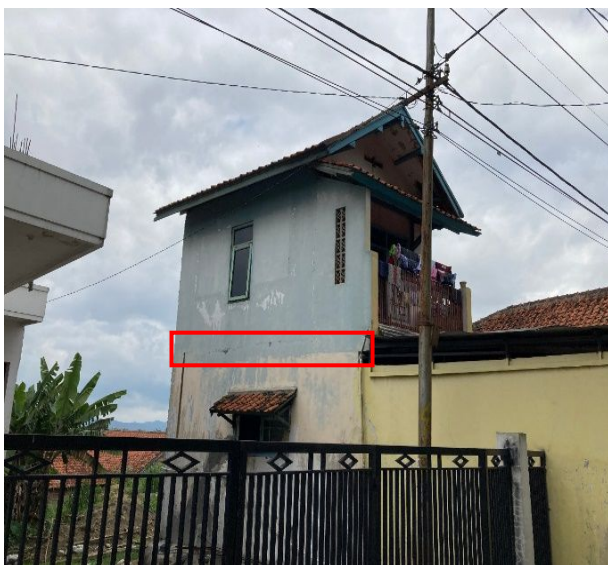
Fig. 5. A building located at CPTu-08 has structural damage. It was marked inside a red box.
