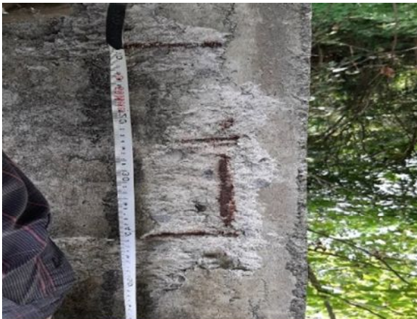
Fig. 2. Steel Reinforcement Corrosion
