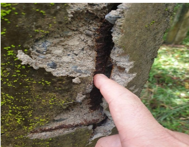
Fig. 4. Porous Concrete and Rusty Steel Reinforcement
