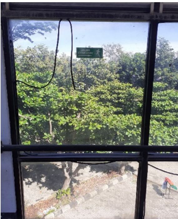
Fig. 13. An example of a misplaced evacuation symbol on Building B, placed on a glass window which is most probably broken firstly on a large earthquake.
