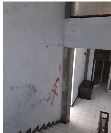
Fig. 10. A large crack in the wall beside the hanging stair, connecting the 2 nd and the 3 rd floor of Building B.
