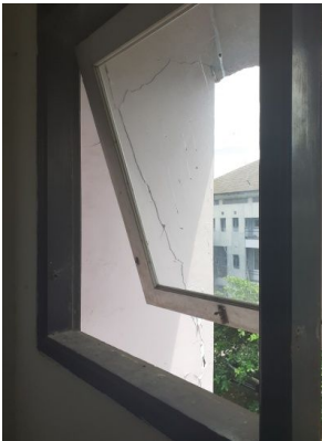
Fig. 6. Cracks in the outside walls of the 3 rd floor of Building A.
