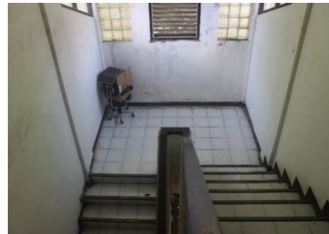
Fig. 15. Inaccessible evacuation route in Building C1, some items are placed in the stair and the next door is locked.
