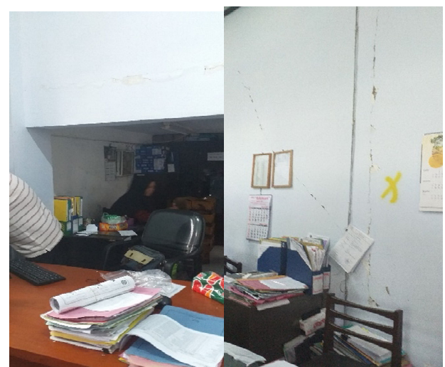
Fig. 4. Staff is working on a narrow place under stairs, and conditions of walls on the 1 st floor of Building A.
