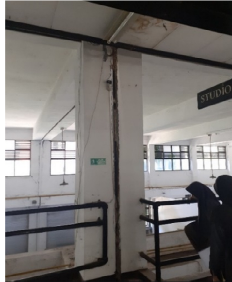
Fig. 9. A large crack between two columns was observed from the 2 nd floor of Building B; the crack is initially from the ground floor.
