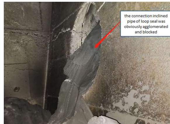
Figure 3. The blockage of loop seal
