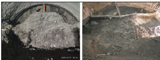
Fig. 8. Excavation face condition from tunnel 6, location measured the rock mass classification from GSI and Q system, left location face mapping 1 and right location face mapping 4
