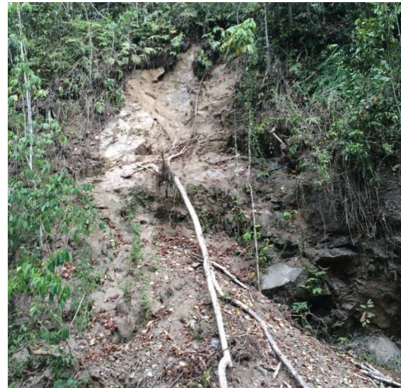
Fig. 8. The Existing slope failure in the study area.
