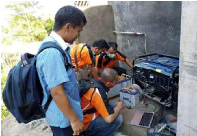
Fig. 2. Biogas conversion generator installation to electricity
