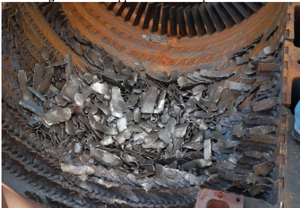
Fig2. Damage degree of compressor blade
