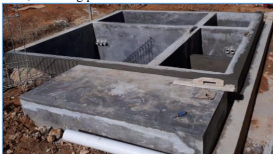
Fig. 4. Cooling water treatment
