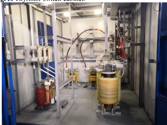
Fig. 6. Power transformer compartment.
