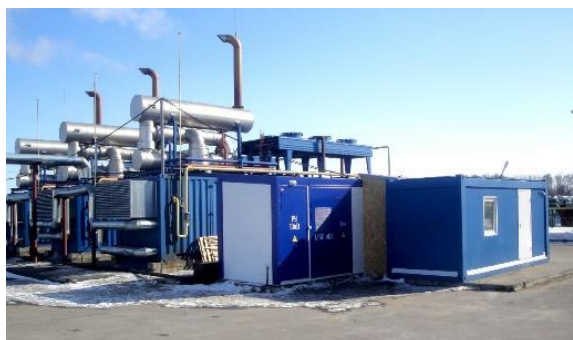
Fig. 1. Experimental power system for testing the combined work of ESS-10-1200-400 and GEG.
