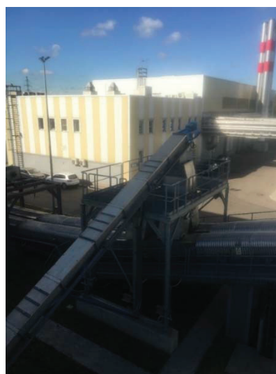
Fig. 4. Dried sludge outlet
