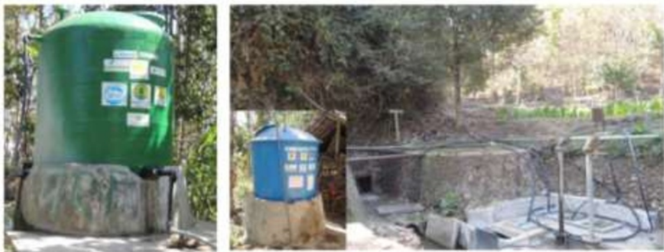
Fig.3. Solar water pumping system in Banyumeneng I hamlet, special region of Jogjakarta (source: kabarhandayani.com)
