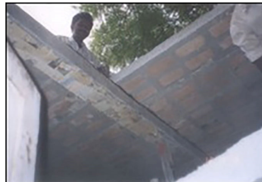
Fig. 9. Details of Reinforced S.C.F Block Slab panel supported on RC joist and wall
