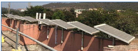
Fig. 3. ASP-12-60W p installed on terrace of SPV Lab
