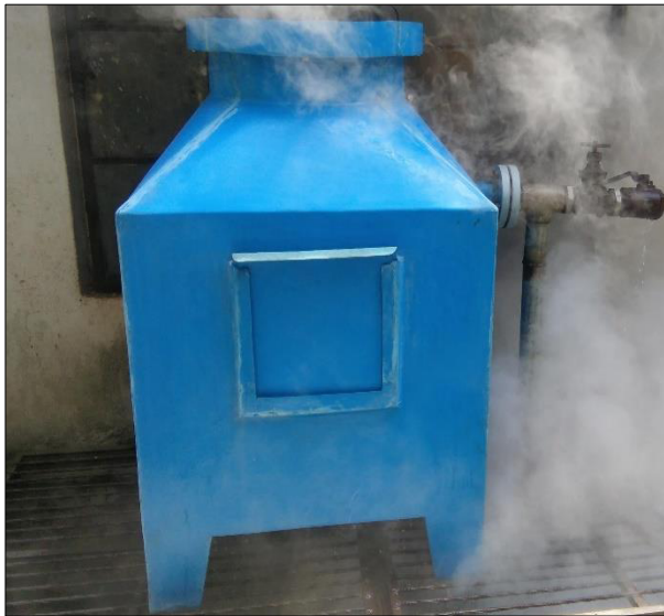
Fig. 3. A packaged type cooling tower; setup
