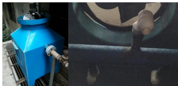
Fig. 1. Packaged type cooling tower and water spraying system inside
