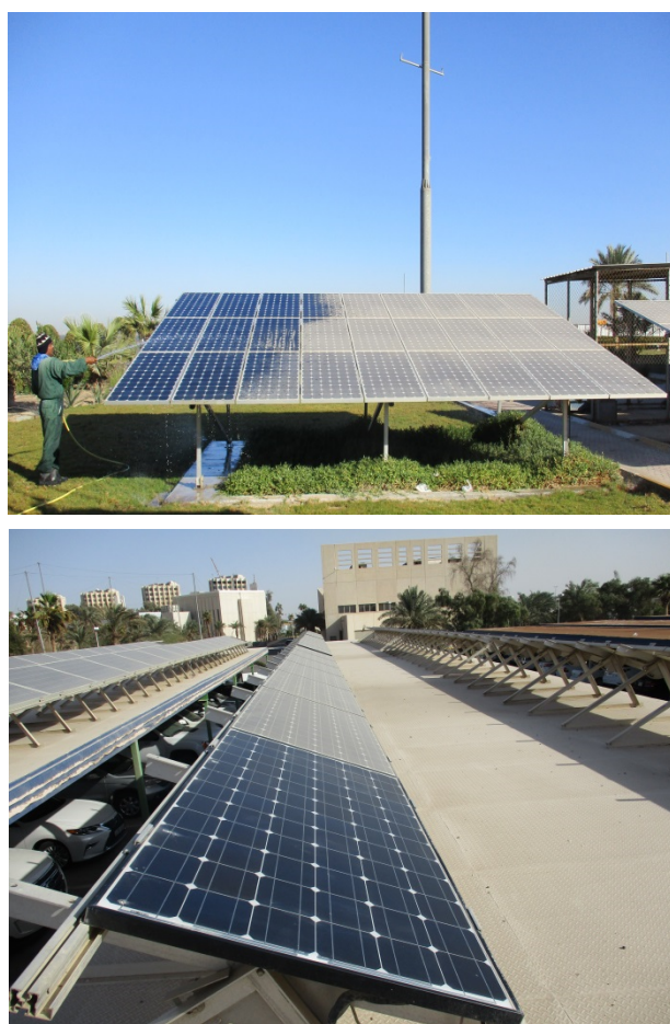
Fig. 3. Dusty solar panels compared to cleaned panels at the KISR.
