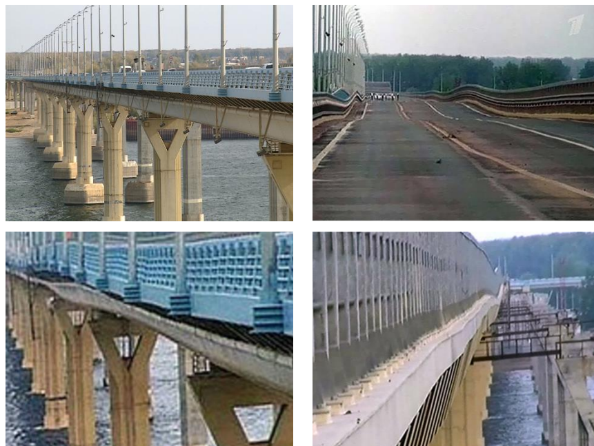
Fig. 2. Volgogradsky Bridge oscillations (the bridge before and during a period of intense oscillations).
