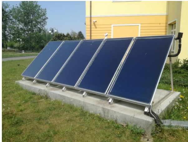
Fig. 2. Diagnosed solar water heating system.
