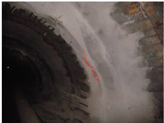
Fig. 15. An ŁP8/V29 steel arch support section covered with shotcrete layer (photo P.Ficek).
