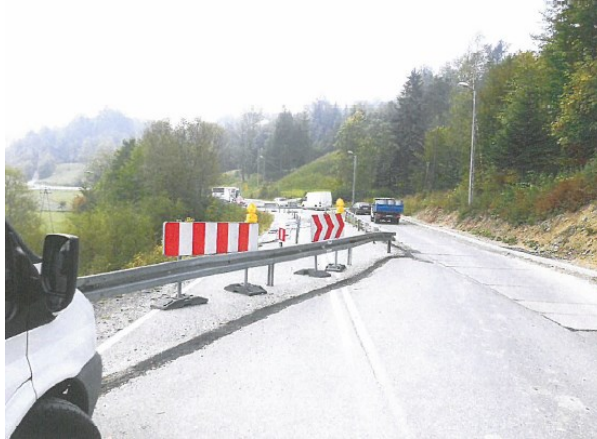
Fig.2. Road surface damage [5].
