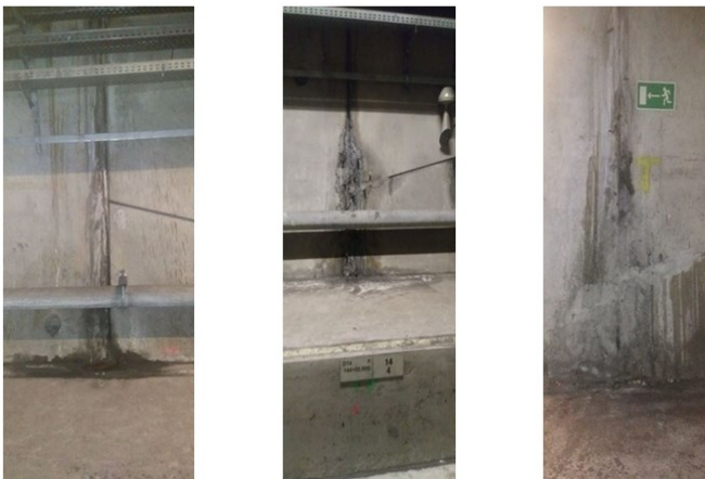
Fig. 4 View of scratches in the metro tunnel and photos of damages of single walls in the tunnel
