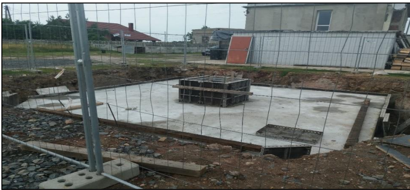
Fig. 5. Reinforced concrete slab with inspection hole securing the Lubichów III shaft barrel.
