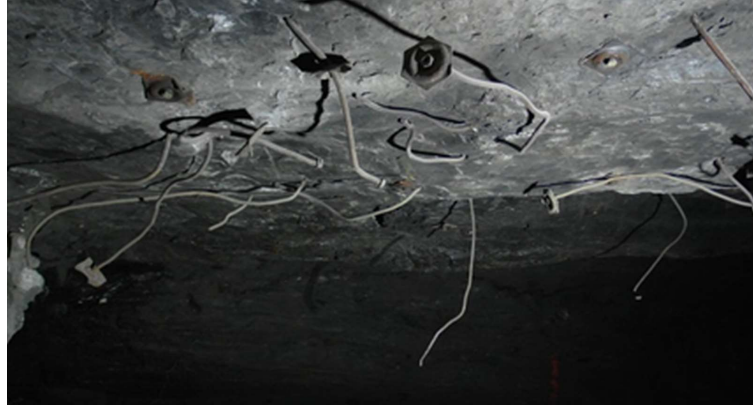
Fig. 1. Result of roof instability occurrence.
